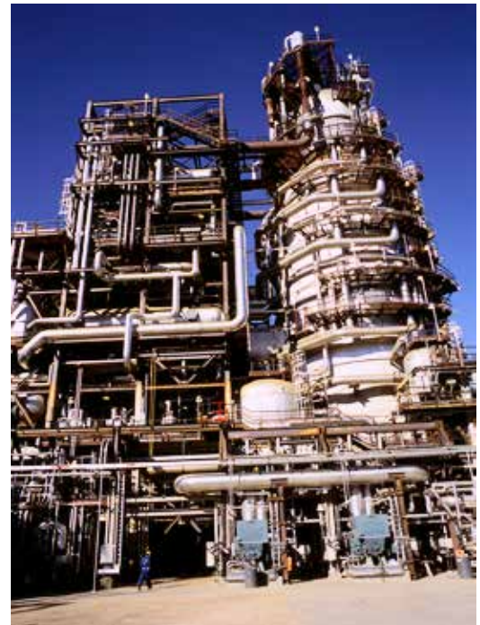
The Shell Scotford Upgrader
