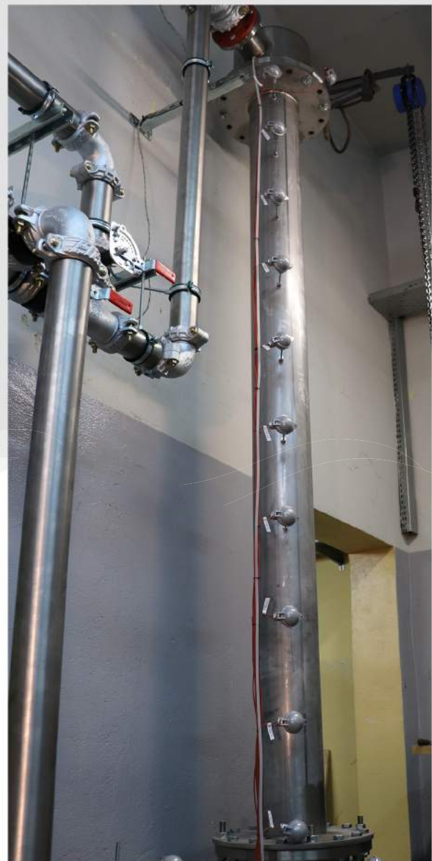
A TES tank without thermal insulation
